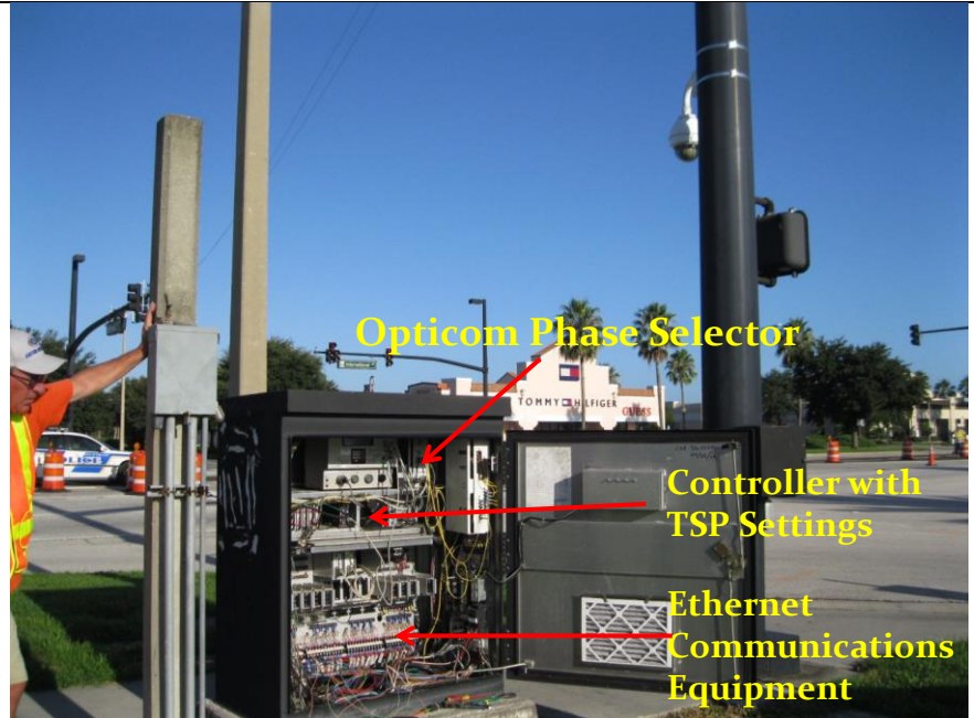
TSP Opticom equipped traffic signal cabinet at Fun Spot in the International Drive corridor in Orlando, Florida; photo credit: Frank Consoli, City of Orlando
